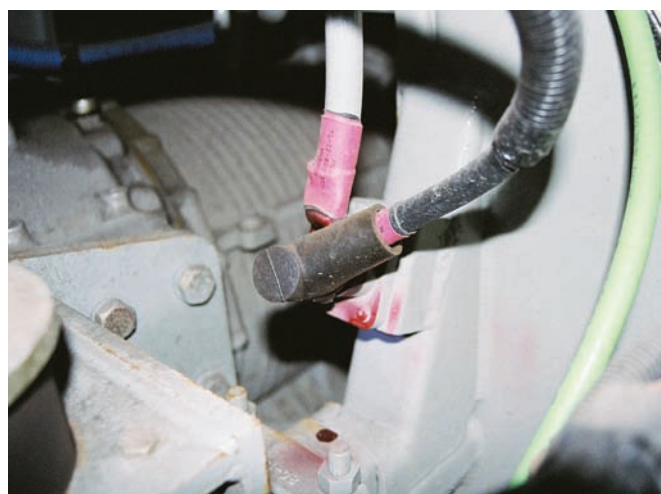
Photo 8B: Bulkhead Connection Bosch T1
