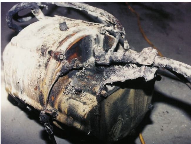
Photo 6B: 50-DN, Result of Failed B+ Stud Insulator
