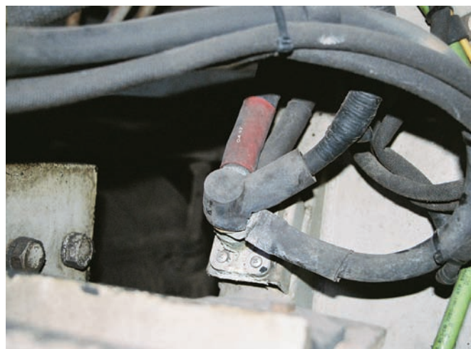
Photo 8A: Bulkhead Connection 50-DN
